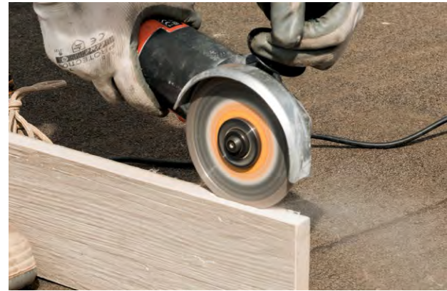
STEP 6 Cut on the edge of the slabs, in order to fit them into the lateral restraint.
