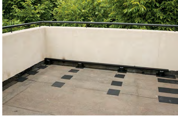
STEP 1 Put the mute mats and the supports into position on the floor (perimeter support must be cut).
